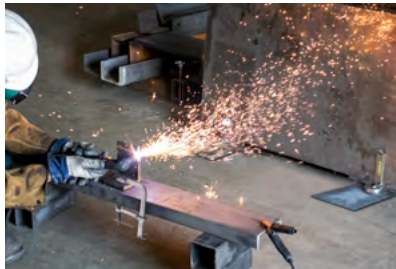
Setup a protective panel wherever needed to protect workers, equipment, and materials from heat, sparks, and slag.
