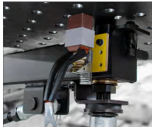
Spring loaded carbon brush grounds rotating plate to stationary grounding point.
